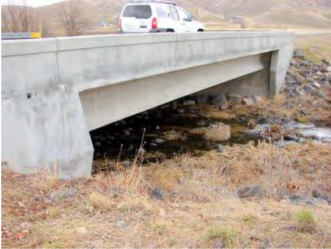
Figure 2. Bridge on Highway 55 near Eagle, Idaho that would provide adequate space for aquatic and terrestrial species. Collisions with deer and other species could be reduced by providing wing-fencing. Photo by Ruediger.
