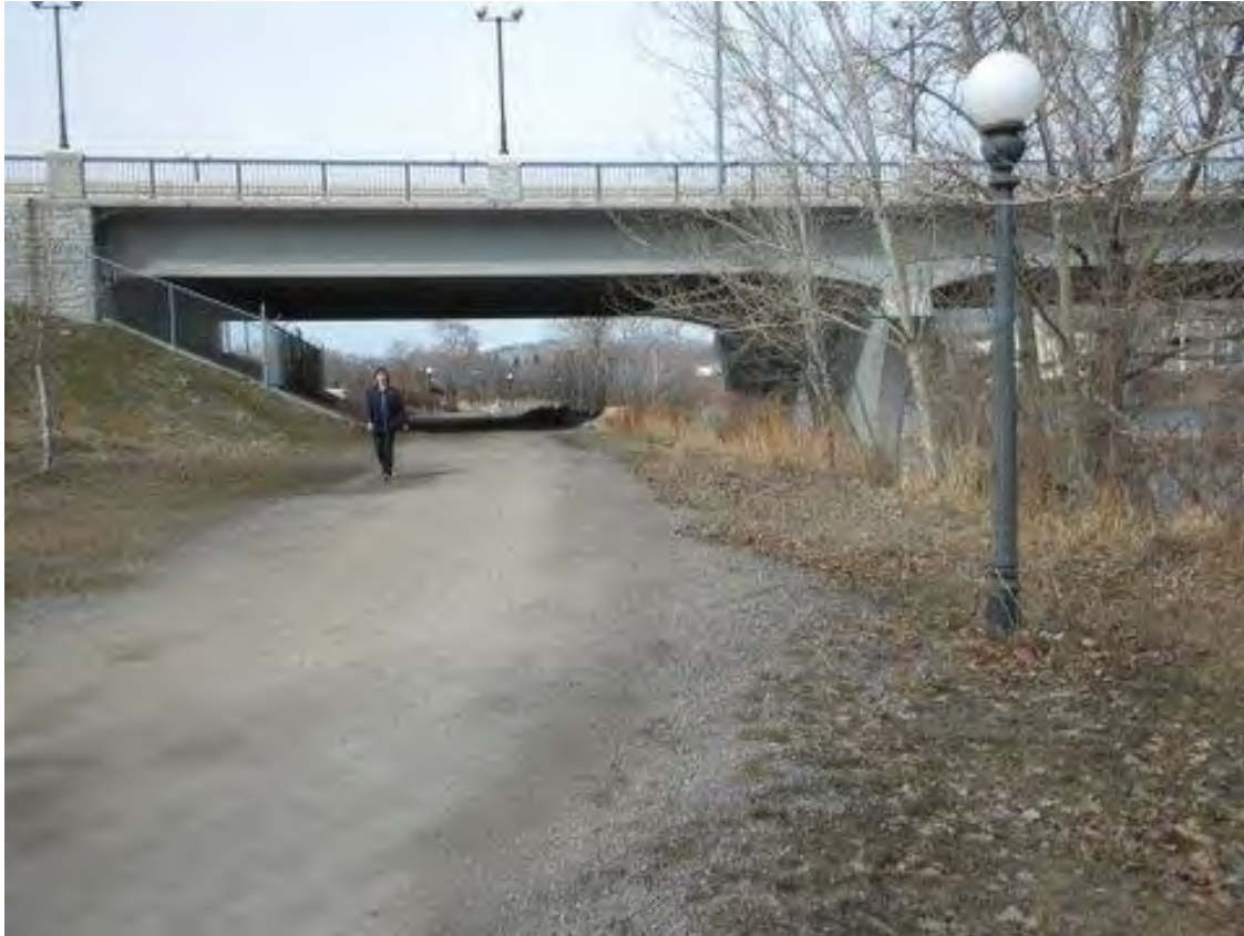
Figure 3. Bridge over the Clark Fork River in Missoula, MT provides adequate space for aquatic and terrestrial species, as well as a hiking trail on each side. Deer and small mammals commonly use this bridge to avoid crossing the busy 4-lane highway. Photo by Ruediger.
